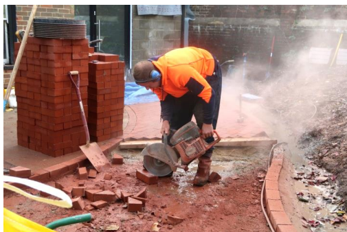
Photo: Laying brick path to new front door. The path is now complete, and can be seen from the Styles Field entrance.
